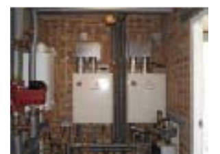
Installation Site - UK (Water Heaters for Commercial Use)
