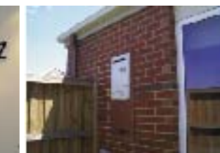
Installation Site - Australia (Water Heater for Residential Use)
