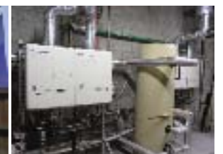
Installation Site - Australia (Water Heaters for Commercial Use)
