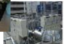
Installation Site - Hong Kong (Commercial manifold system)
