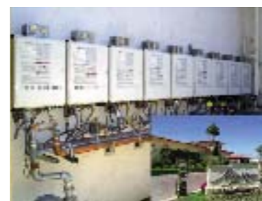
Installation Site - USA (Commercial manifold system)
