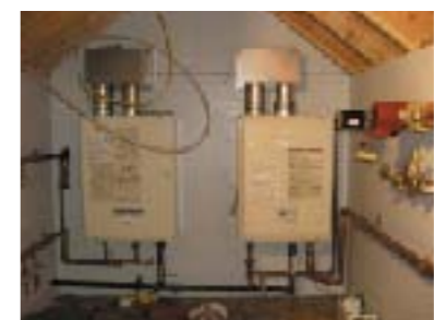
Installation Site - USA (Water heater and space heater)
